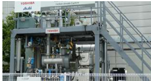
Experimental CO 2 Separation and Recovery Equipment
