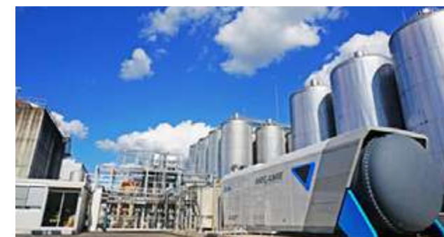
System to Generate Power from Biomethane-Gas-powered Fuel Cells
