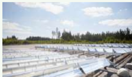
Solar collectors at Bari Brewery in Italy
