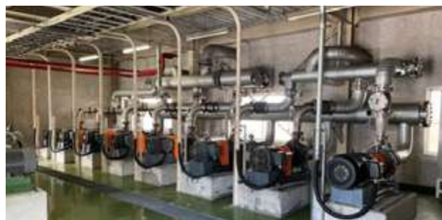
Water treatment facility (Nagoya Brewery)
