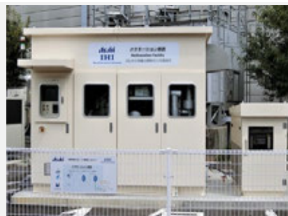
A methanation device aimed at effective use of CO 2
